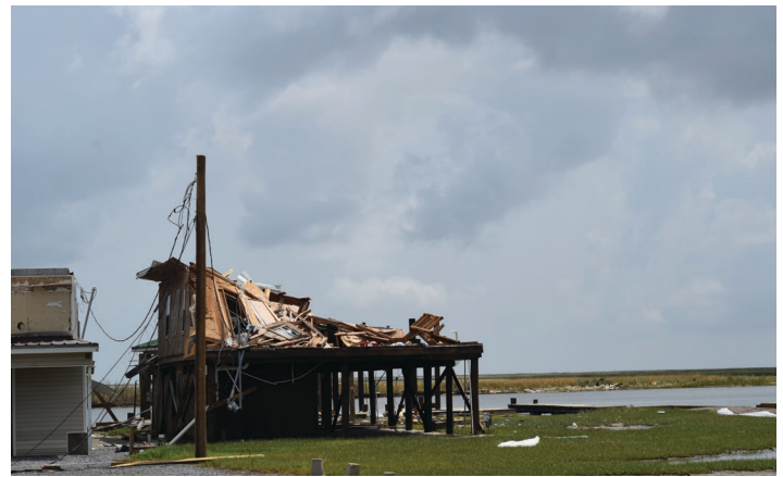
Figure 1. Building collapse near Cocodrie (Photo by Brandon Rittelmeyer).
