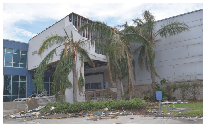
Figure 3. Cladding damage to South Lafourche High School. 1
