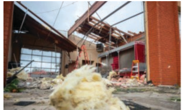
Figure 2. Damage to Little Calliou Volunteer Fire Department Station in Chauvin 1
