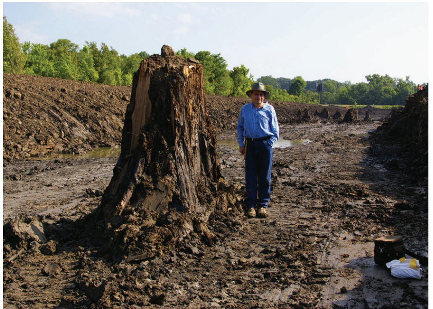
Figure 2. Photograph of the author standing by an upright buried cypress stump uncovered by excavation adjacent to BREC Burbank Soccer Complex and Burbank Drive, Baton Rouge, Louisiana.
